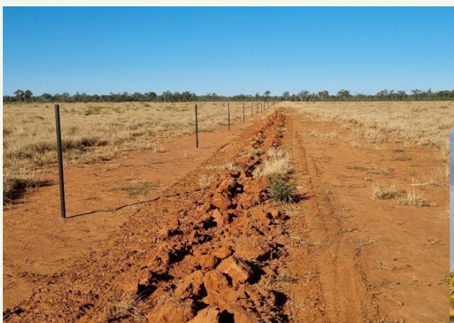
Poly pipe is buried parallel to a new fence line and distributed to troughs located 1km apart.
