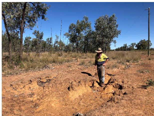
Photo. Eroded track/road.
